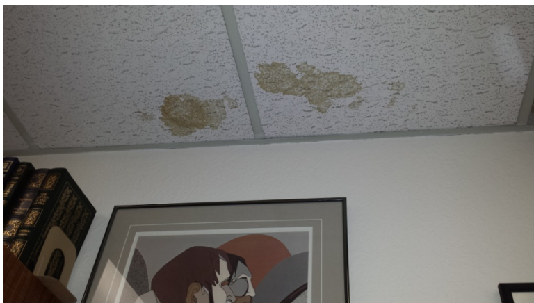
Figure 13 Water damage to second floor ceiling
