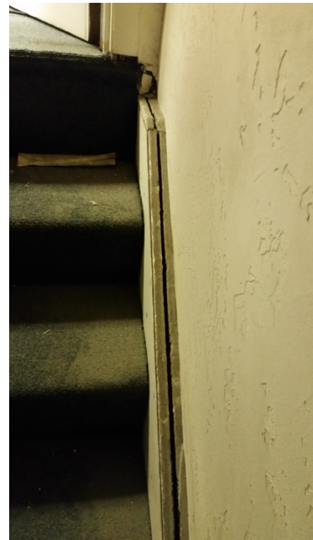
Figure 3 Separation at west side of stair
