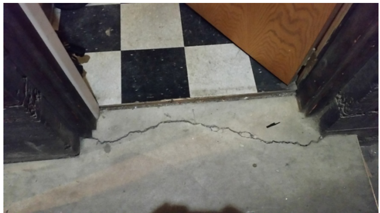
Figure 9 Crack in slab at east side of storeroom.
