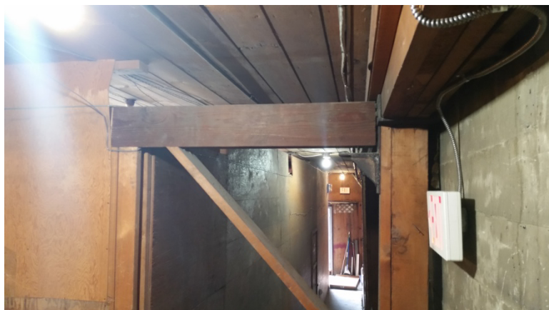
Figure 4 Gap at settled column
