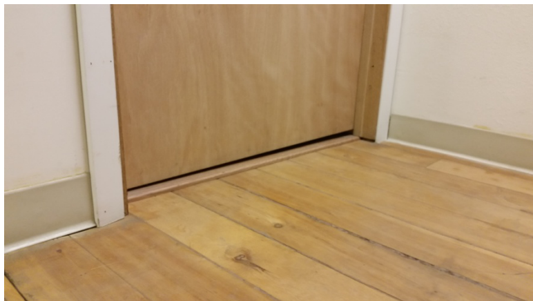
Figure 7 Slope in floor at door sill
