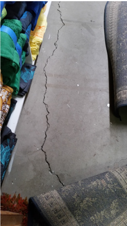
Figure 10 Crack in slab in storeroom
