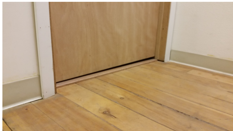
Figure 7 Slope in floor at door sill
