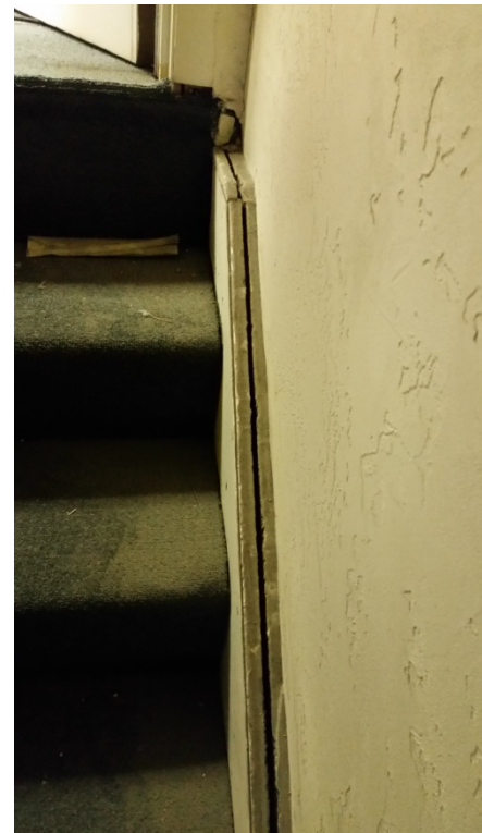
Figure 3 Separation at west side of stair
