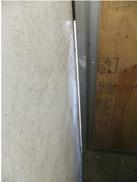
Figure 2 Separation at door frame at base of stair
