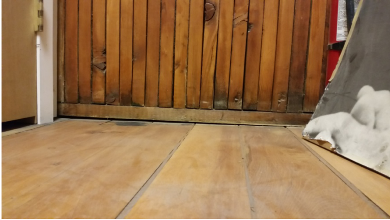
Figure 8 Slope of floor at interior wall
