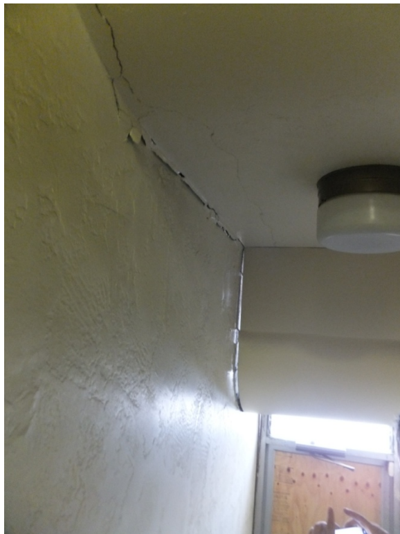
Figure 1 Separation at west wall of stair
